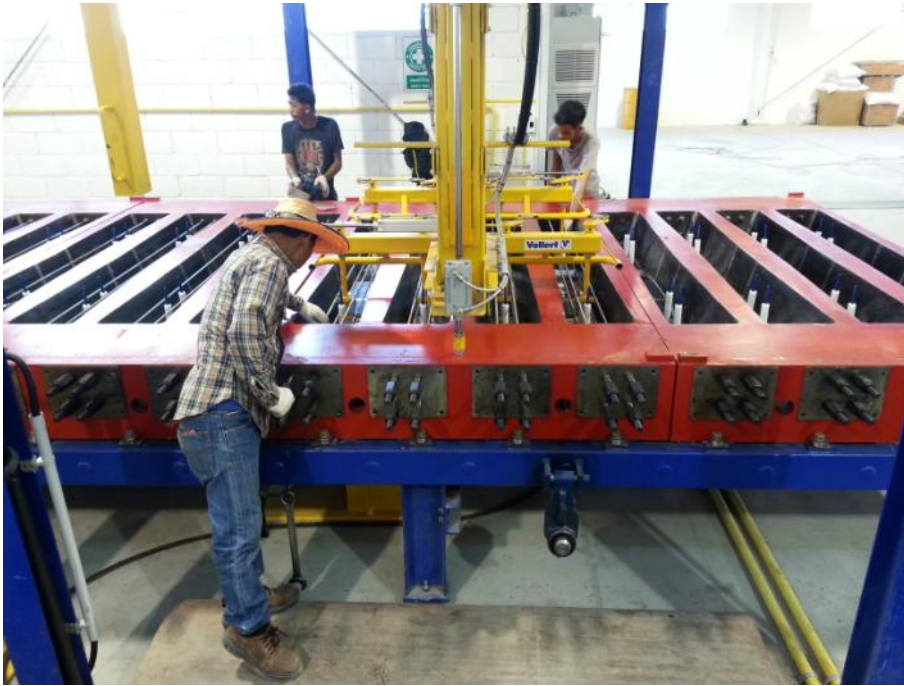
Fig. 3: First of all the individual wires are manually fastened in the mould with the pre-mounted tensioning and anchor bolts.
