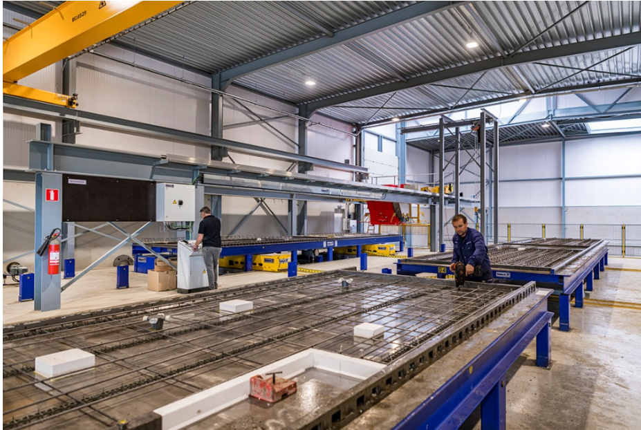
Image 1 The Belgian building materials specialist Daerden expands its capacities in the production of serially prefabricated concrete semi-finished parts.
