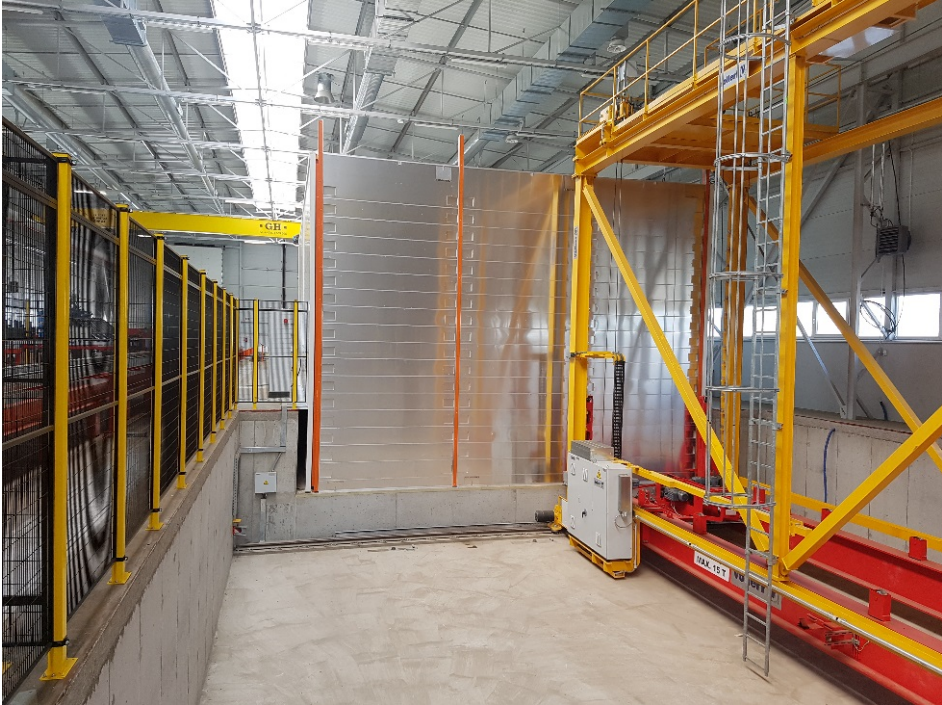
Image 5 The 17-level shelf towers are controlled by means of a centrally installed, floor-mounted Vario STORE storage retrieval machine.
