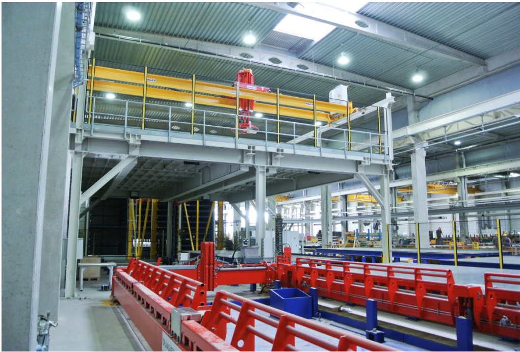
Fig. 5: For high quality of the exposed concrete of the solid concrete parts, these parts are transported onwards to a smoothing station on a 2 nd level
