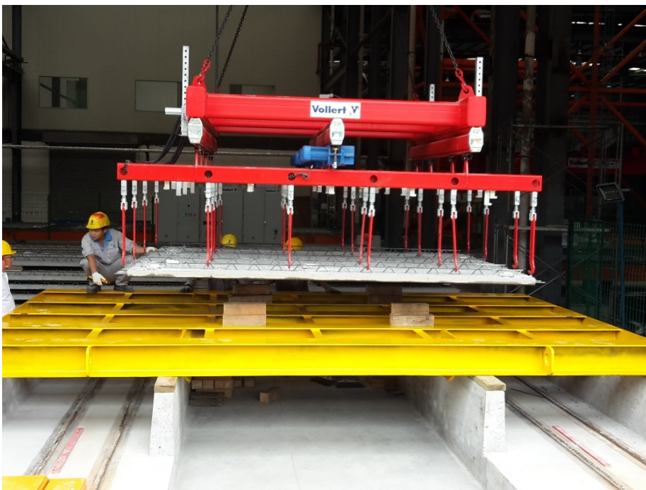
Fig. 8: Floor slabs are provided horizontally in transport-capable stacks with a lifting device
