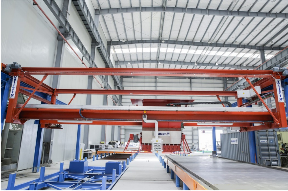
Fig. 3: Precise application of the concrete by a modern SMART CAST automatic concrete distributor
