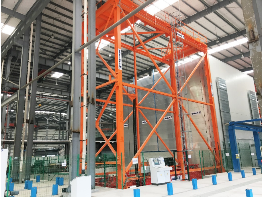
Fig. 5: The insulated and heated shelf towers of the curing chamber are controlled via the VARIO STORE storage retrieval machine
