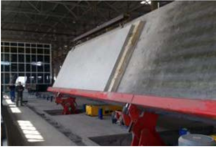
Fig. 7: The solid and sandwich elements are lifted off vertically by a high-performance tilting station
