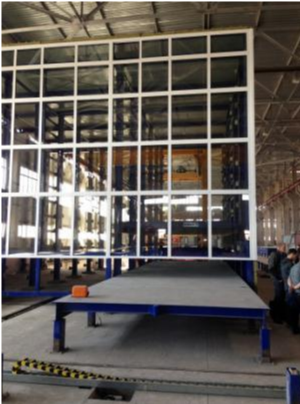
Fig. 6: The heated hardening chamber consists of rack towers clad with thermally insulating glass
